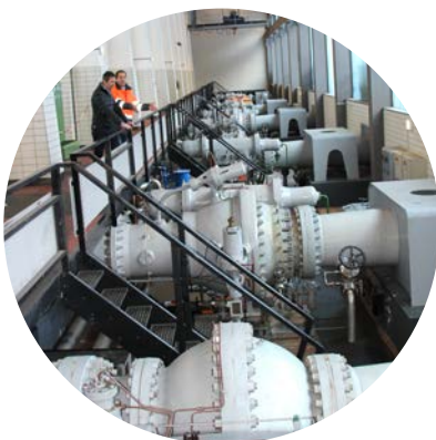
POWERBANK. Inside the turbine room of the ÖBB power plant at Enzingerboden
