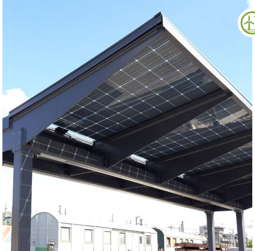
PHOTOVOLTAIC ELEMENTS serve as the roof of a bike shelter
