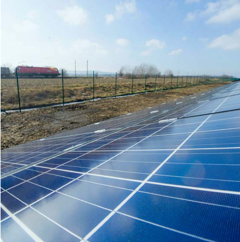
SOLAR POWER. The world's first photovoltaic system for traction in Wilfleinsdorf.
